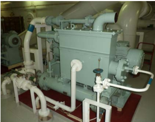
Gambar 3. Vacuum pump (LNG/C Golar Mazo document)
